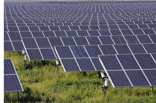
A solar farm
