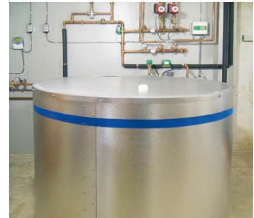
Hot water storage tank in the basement of a smart house
